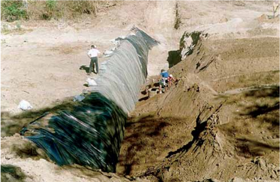
Photo 10 – Aspect of the Trench of an Underground Dam, Showing in the Center, the Piezometric Well Foundation Source: João Bosco de Oliveira.
